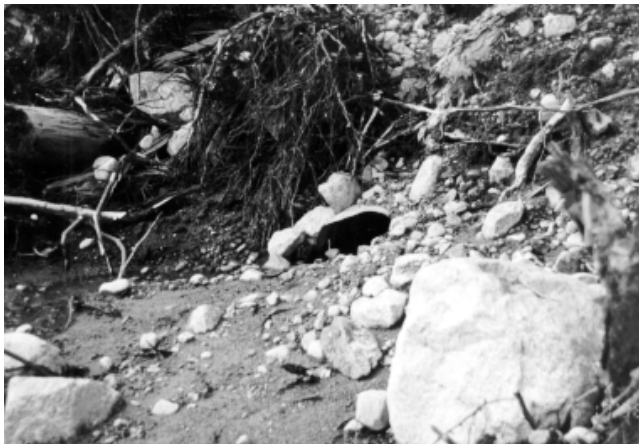
This stream crossing in Solski Township had a seriously blocked culvert, resulting in flooding and siltation.
